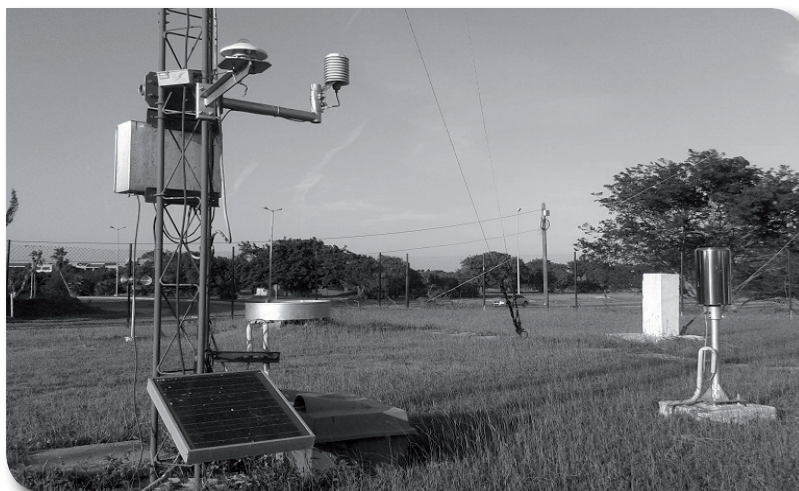
Automated meteorological station
